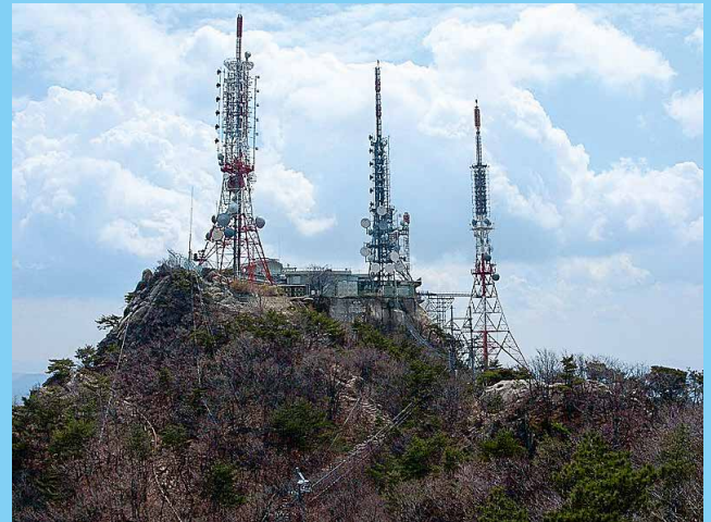
The KBS antenna tower (left) is used to broadcast the world's first terrestrial 4K programs.
